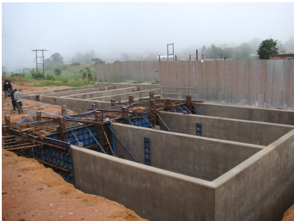
National Water Development Program: Water treatment plant under construction for Northern Region Water Board
